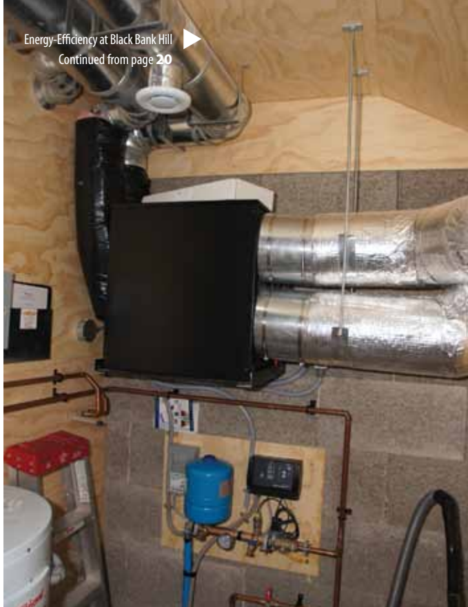
▲ Located near the pantry, the mechanical room houses an energy recovery ventilator which exhausts hot, stale air from the air-tight house and supplies cool, fresh air. While making this exchange, heat and moisture from the stale air is transferred to the fresh air, reducing energy waste with a 95 per cent heat recovery rate.
